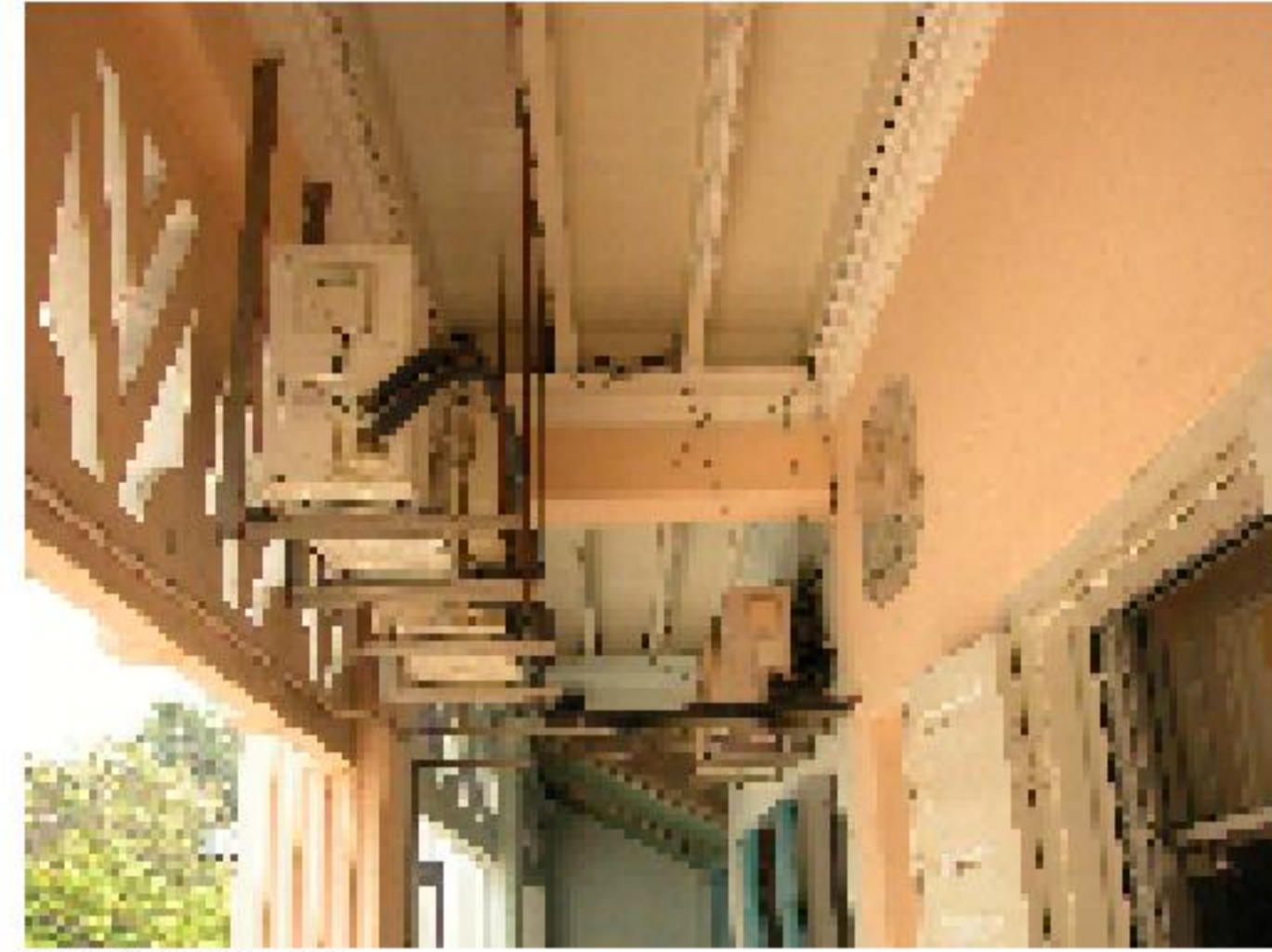
Wall placed air compressor
